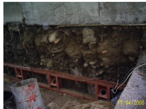
Fig. 14. A fragment of a wall made of pillars made by jet cementation in blocked soils for fencing a pit for a high-rise building near the Romashka store in Minsk
