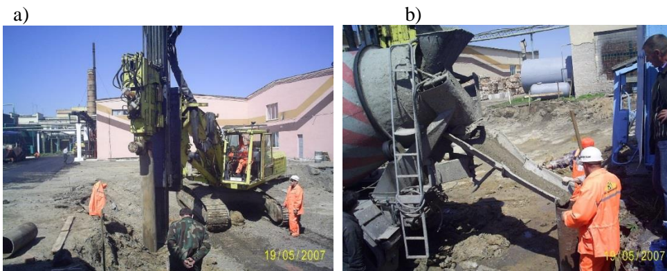
a - immersion of a casing pipe with a lost tip into a water-saturated soil using an ABI machine with a vibrator on a guide rod; b - concreting of the pile shaft
