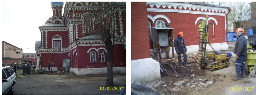
Fig. 12. Work on strengthening the soils at the base of the pile foundations of the Holy Ascension Church in Borisov with the help of drilling piles (on the lower the image shows a small-sized drilling rig in the process of drilling wells)
