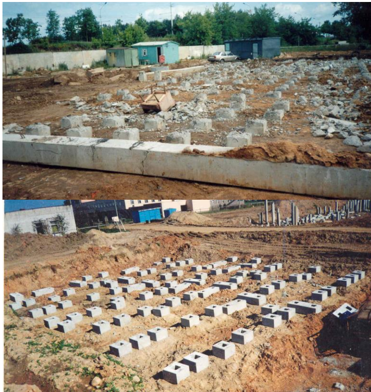
Fig.4. Pile field after cutting down the upper sections of piles and after laying prefabricated headrests on them
