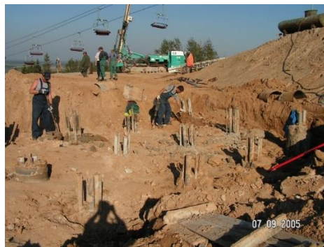
Fig. 13. Piles made using jet technology for the end support on the slope of the ski slope in Silichi
