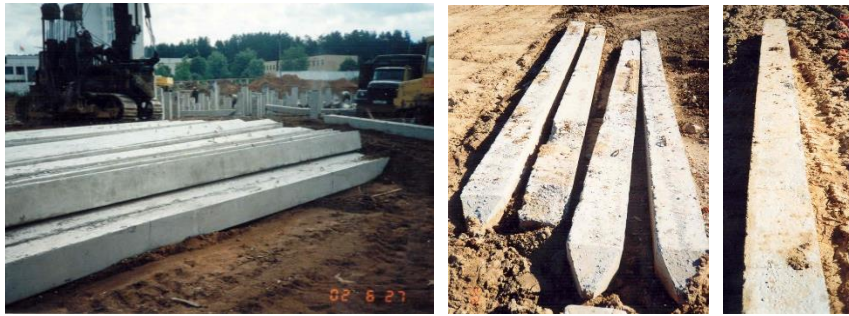
Fig.3. Defects in pile trunks during incorrect laying on the soil surface
